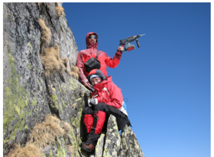
Fig. 7. Instalation of crack extensometer in rock walls from Retezat Mountains (Photo R. Popescu).
