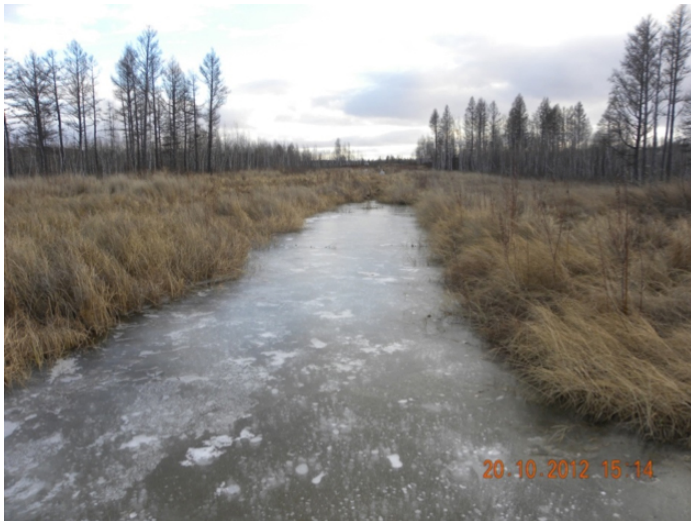
Figure 1. Ponding of deep water in the subsided right-of-way zone along the China-Russia Crude Oil Pipeline.
